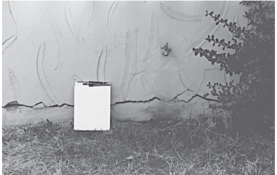
Stresses on buildings due to minor earthquakes, wind, snow, or even changes in loads, such as furniture, large numbers of people, remodeling, adding/removing walls, counters, etc., can cause building elements to shift or warp over long periods of time.
